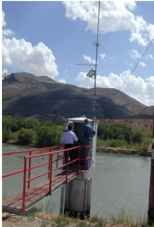
Telemetry Gage Station
